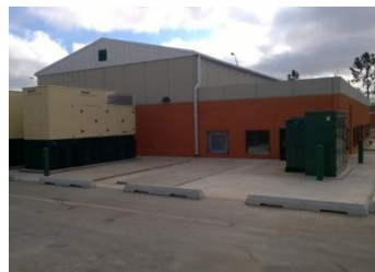
PRIMARY DATA CENTER
