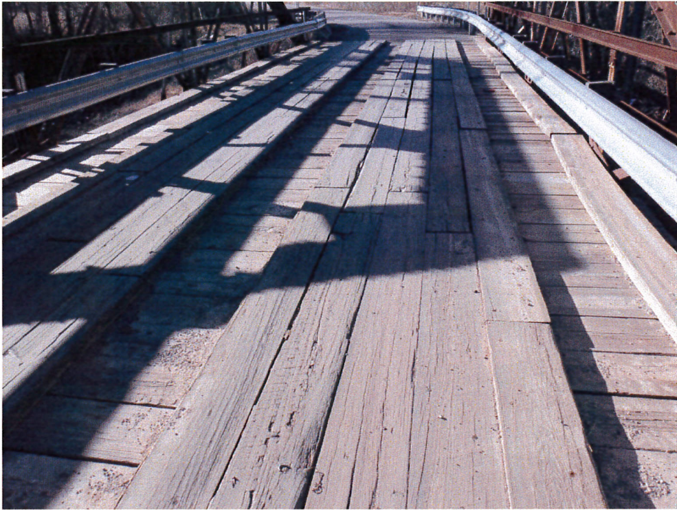
Figure 5: Typical Cracking in Runners
