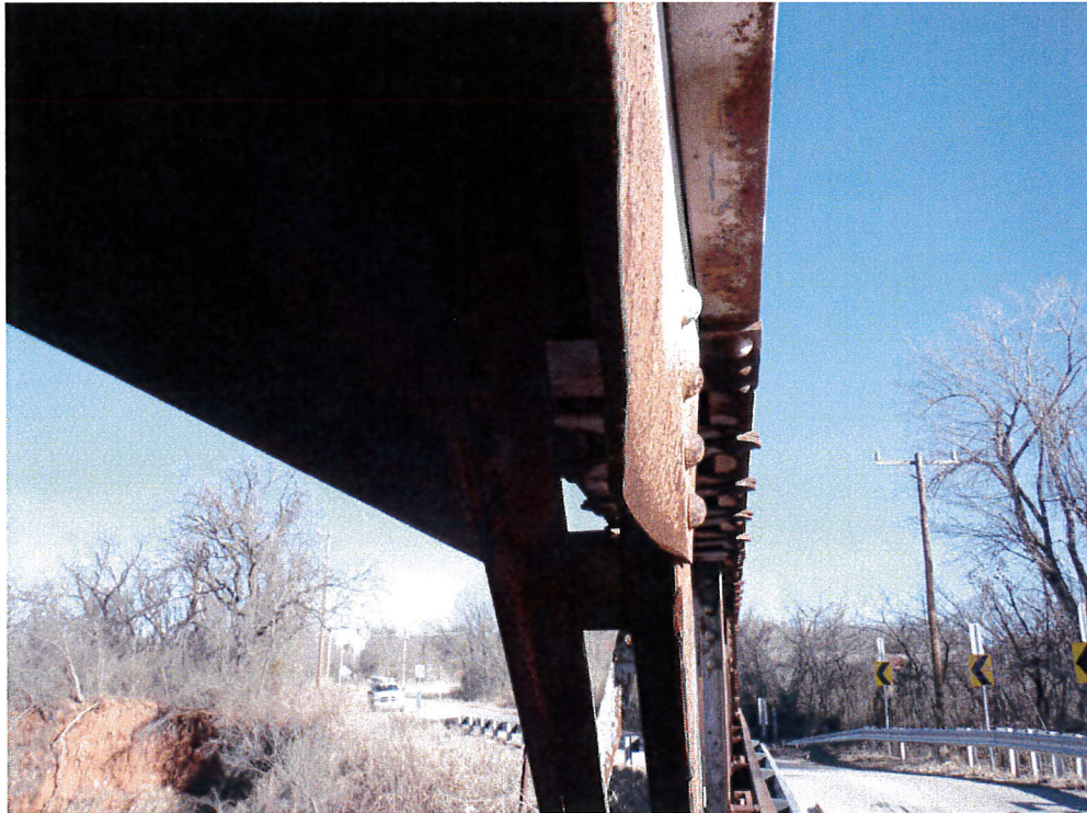
Figure 11: Warped Gusset Plate at U3, West Truss (From previous impact damage)
