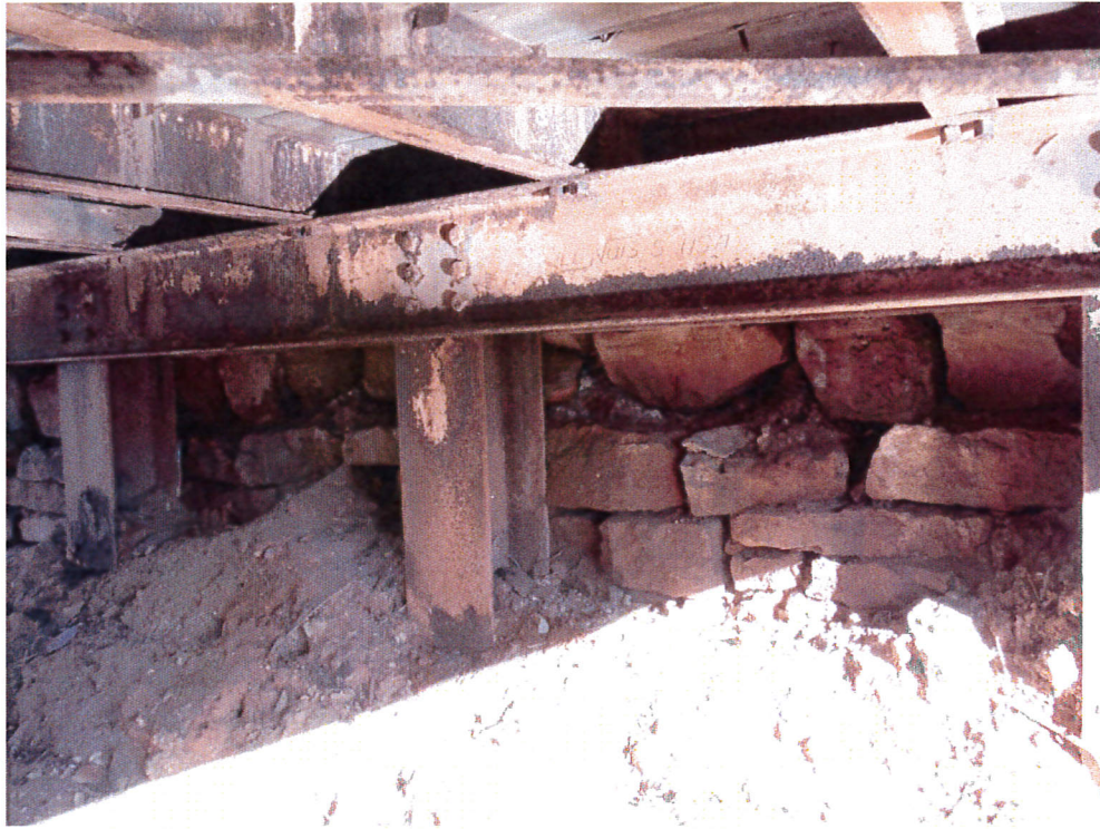
Figure 13: Typical Corrosion of Steel Cap North Abutment
