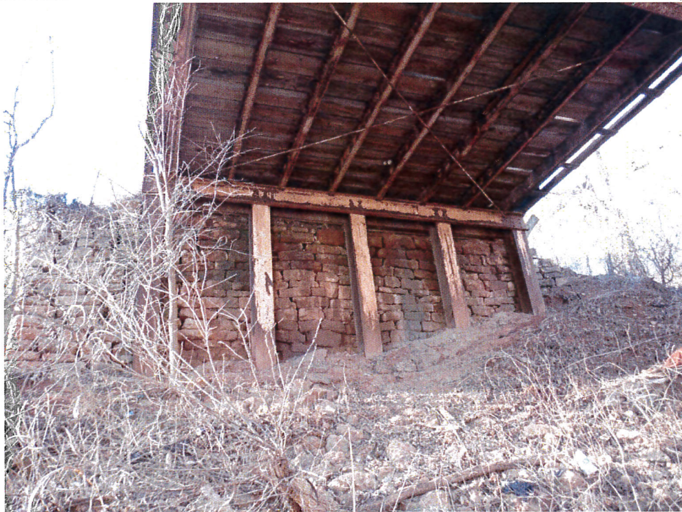
Figure 15: Stone Masonry with Open Gaps South Abutment
