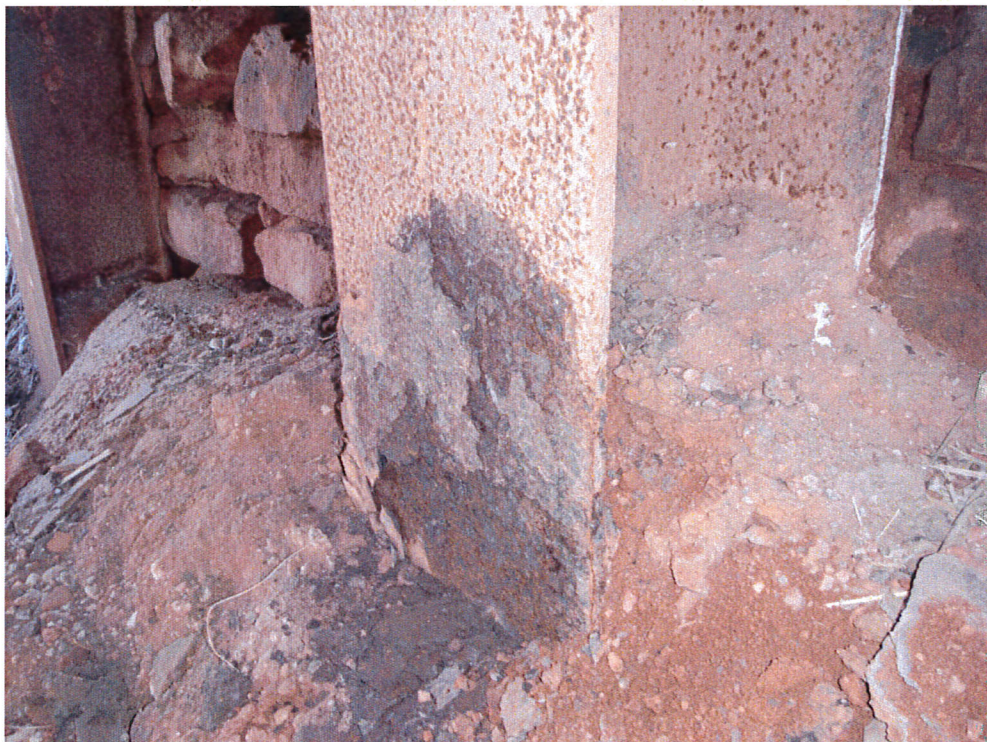
Figure 14: Typical up to 15% Section Loss of Pile 2, South Abutment
