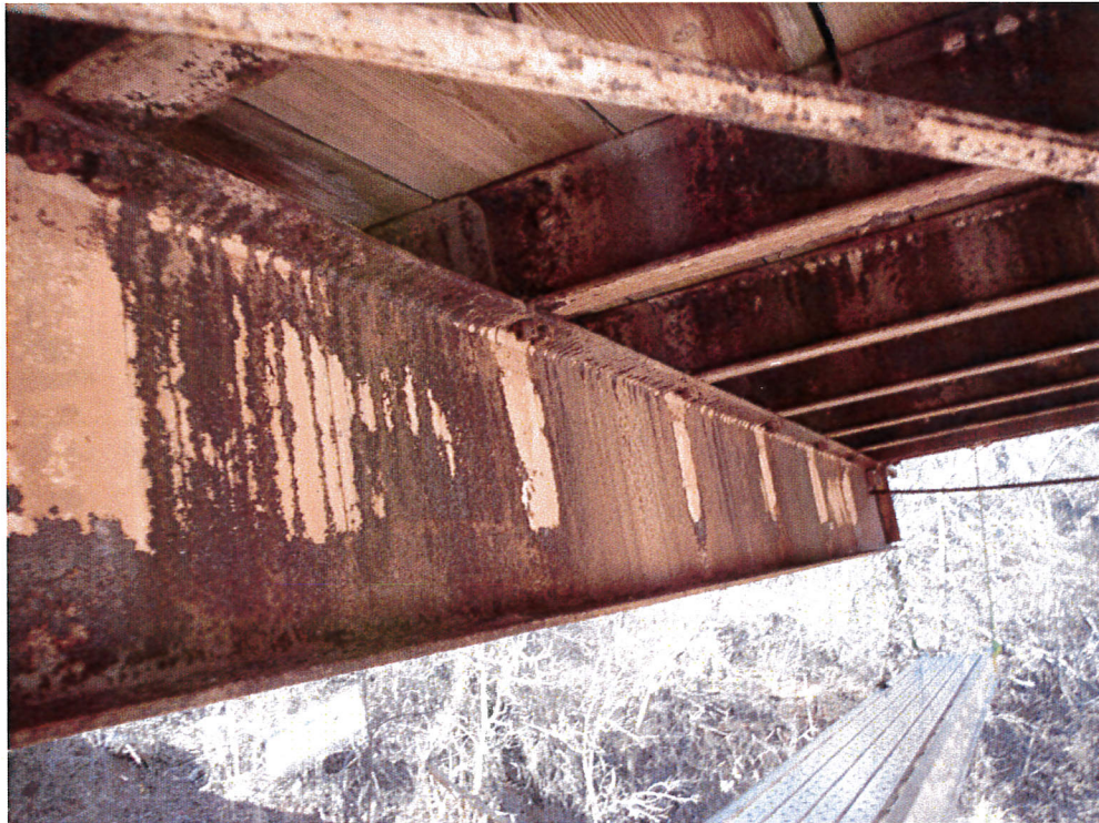
Figure 7: Floor Beam 4 Overall Surface Corrosion
