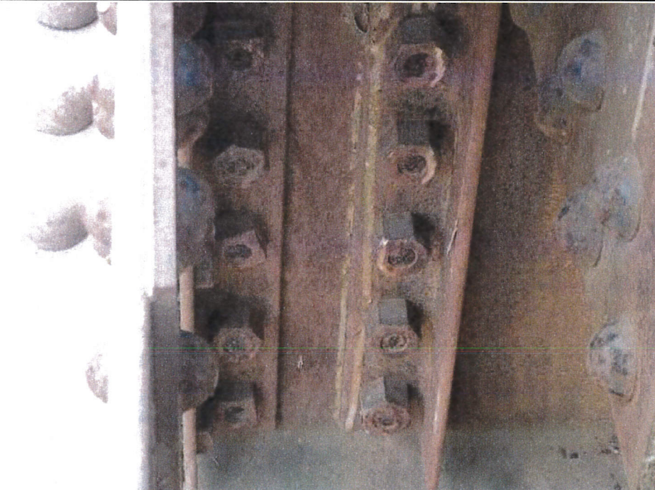
Photograph 8 - Looking south at east truss L2, bolted connection of vertical to floor beam. Note: Bolt shanks are not long enough to extend through nut. Typical to all floor beam connections.
