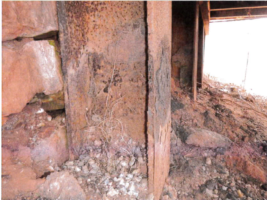
Photograph 13 - Looking northeast at southwest corner of pile 2 at north abutment. Note: Section loss up to 1/8-inch deep on south flange for approximately a 4-inch height of the steel bent.
