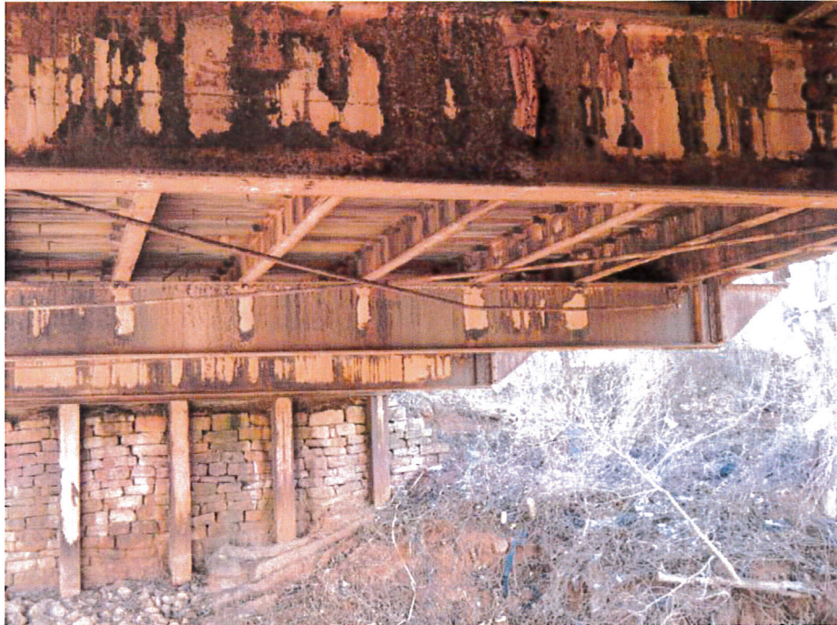
Photograph 9 - Looking southwest at lower lateral bracing bar between floor beams 3 and 5 between stringers 3 and 4. Note: Bar is bent down, no change from last inspection.
