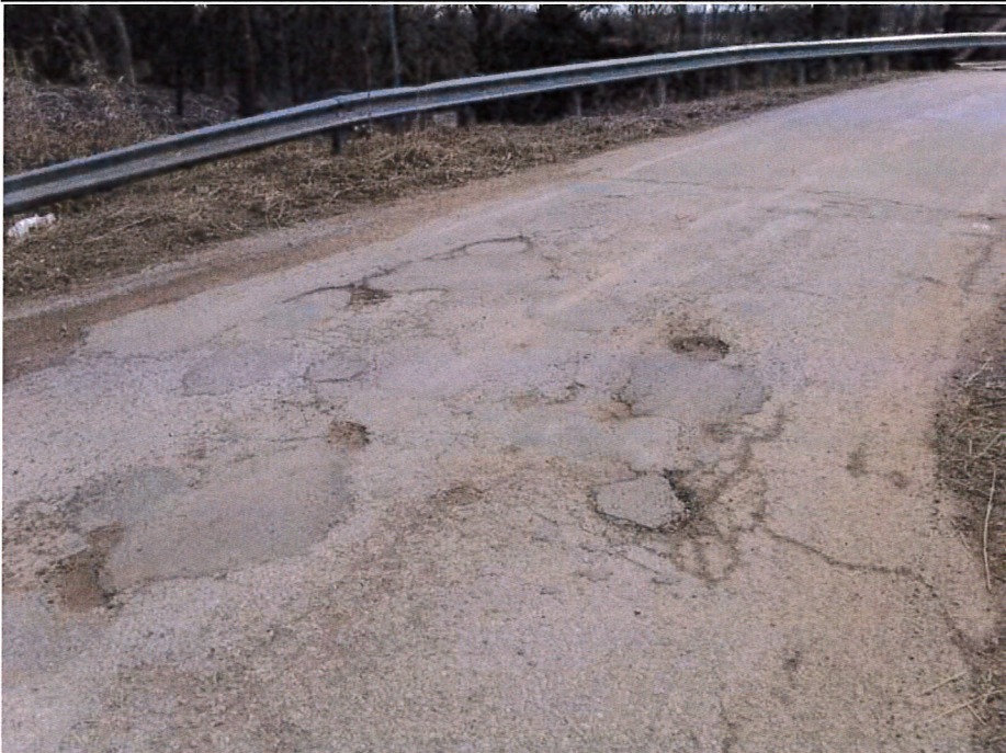
Photograph 18 - Looking northwest approximately 100 feet north of the bridge. Note: Extensive patches and potholes exist in the south approach roadway.
