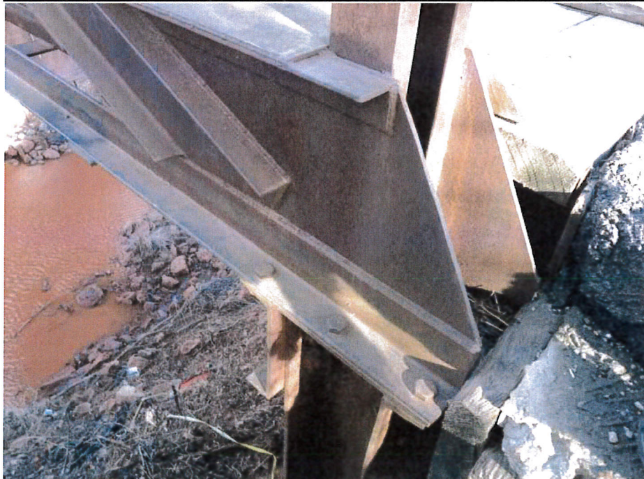
Photograph 14 - Looking northeast at L0, west truss. Note: The steel plate bearings exhibit surface corrosion with light amounts of minor pitting.
