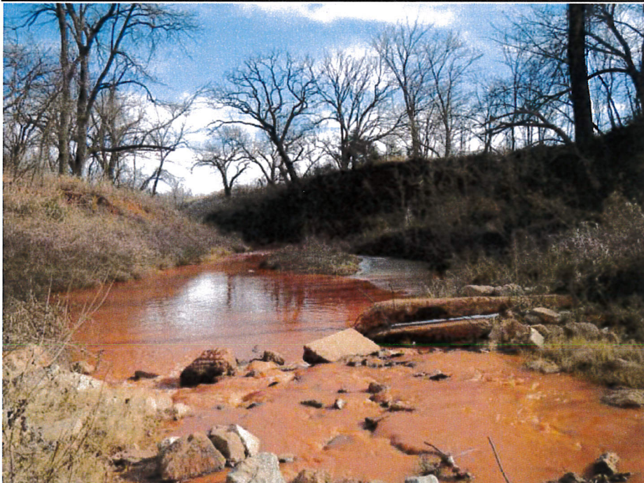
Photograph 16 - Looking east downstream of bridge. Note: channel slopes are sloughing heavily and washing out due to channel scour.
