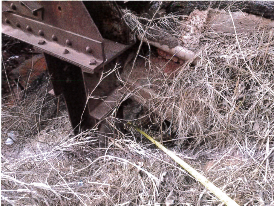
Photograph 17 - Looking west at the north approach roadway which is undermined up to 2 feet at the northeast corner of the bridge up due to erosion.
