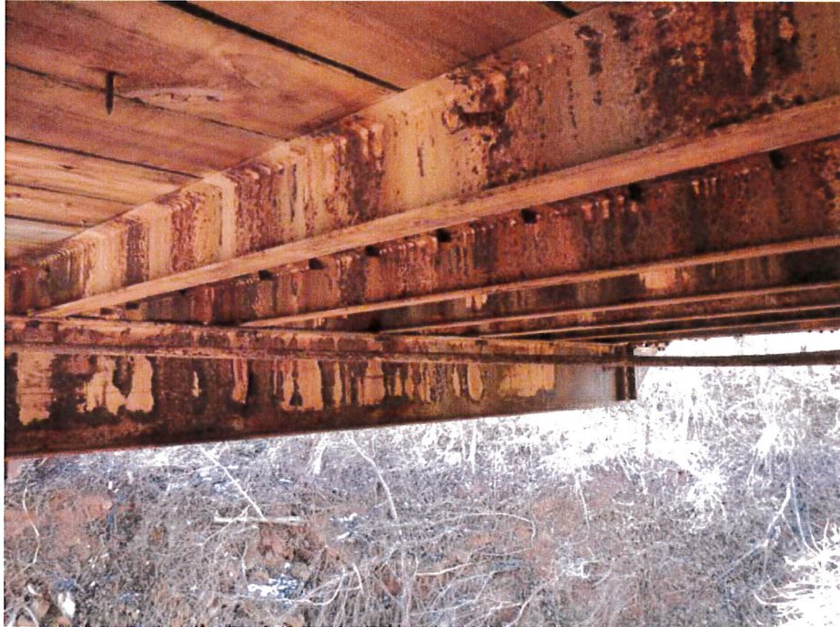
Photograph 11 - Looking southwest at overall typical condition of steel floor system with corrosion and failing paint throughout.
