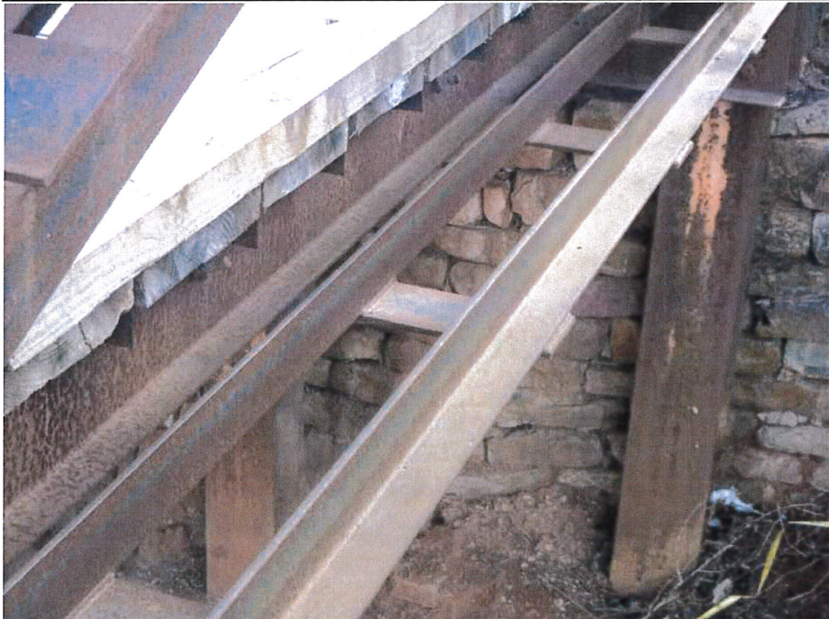
Photograph 10 - Looking southeast at west truss, lower chord. Note: L0L2 has been replaced with batten plates welded to lower chord in this section.
