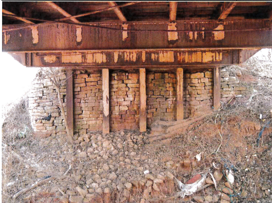
Photograph 12 - Looking south at overall view of north abutment breastwall. Note: Masonry blocks have no mortar between stones throughout abutment wall.
