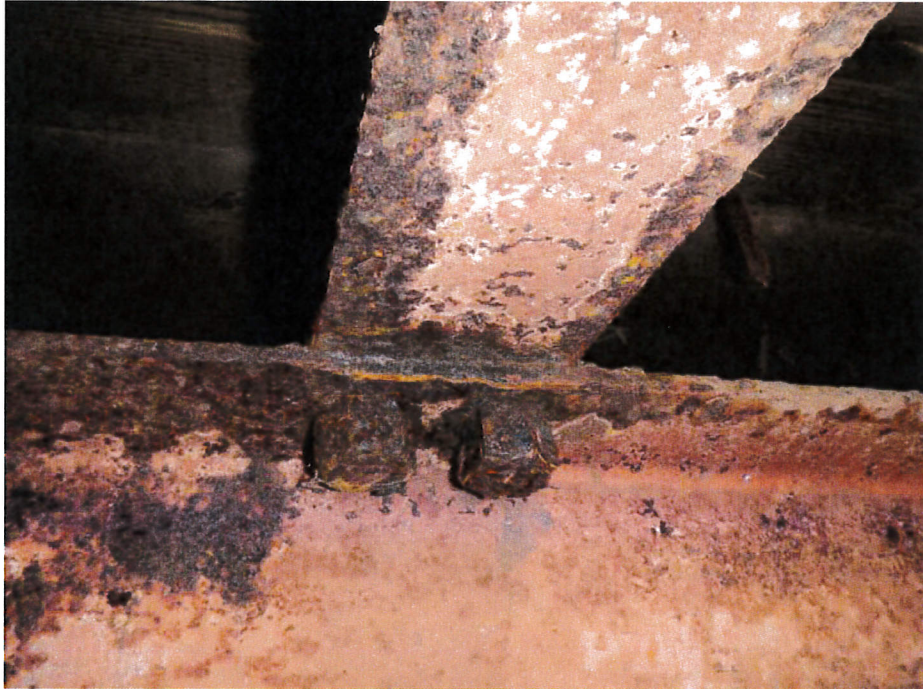
Photograph 7 - Looking north at the stringer 5 bottom flange connection to the north abutment pile cap. Note: Up to 1/4-inch loss to bottom flange.
