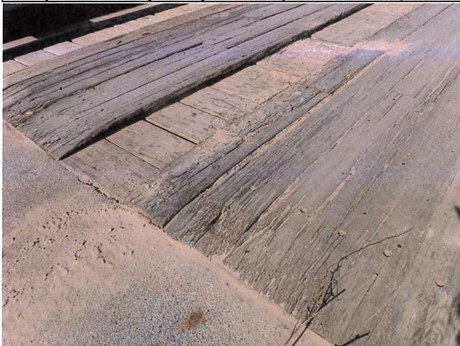
Photograph 6 - Looking north at the south end of the bridge deck. Note: The longitudinal runners have checks and splits along their length, which appear heavier towards the ends of the bridge.
