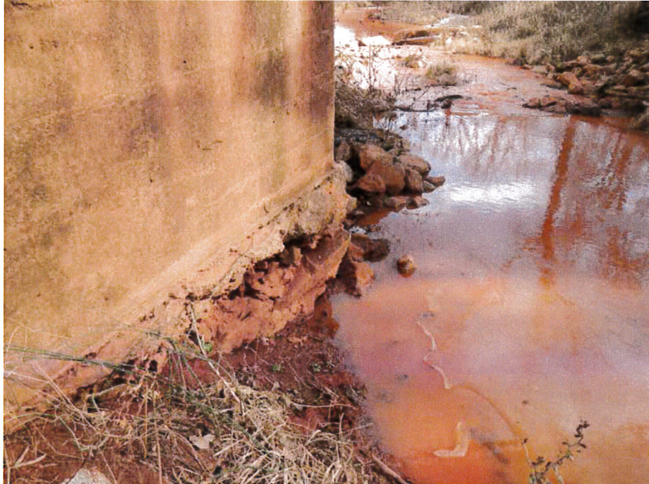
Photograph 15 - Looking southeast at base of the old concrete abutment in front of the current north abutment. Note: east end of old abutment has rock foundation exposed.
