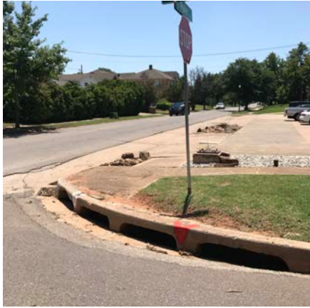
Figure 19. Large storm drains on Walker Avenue create safety hazards.
