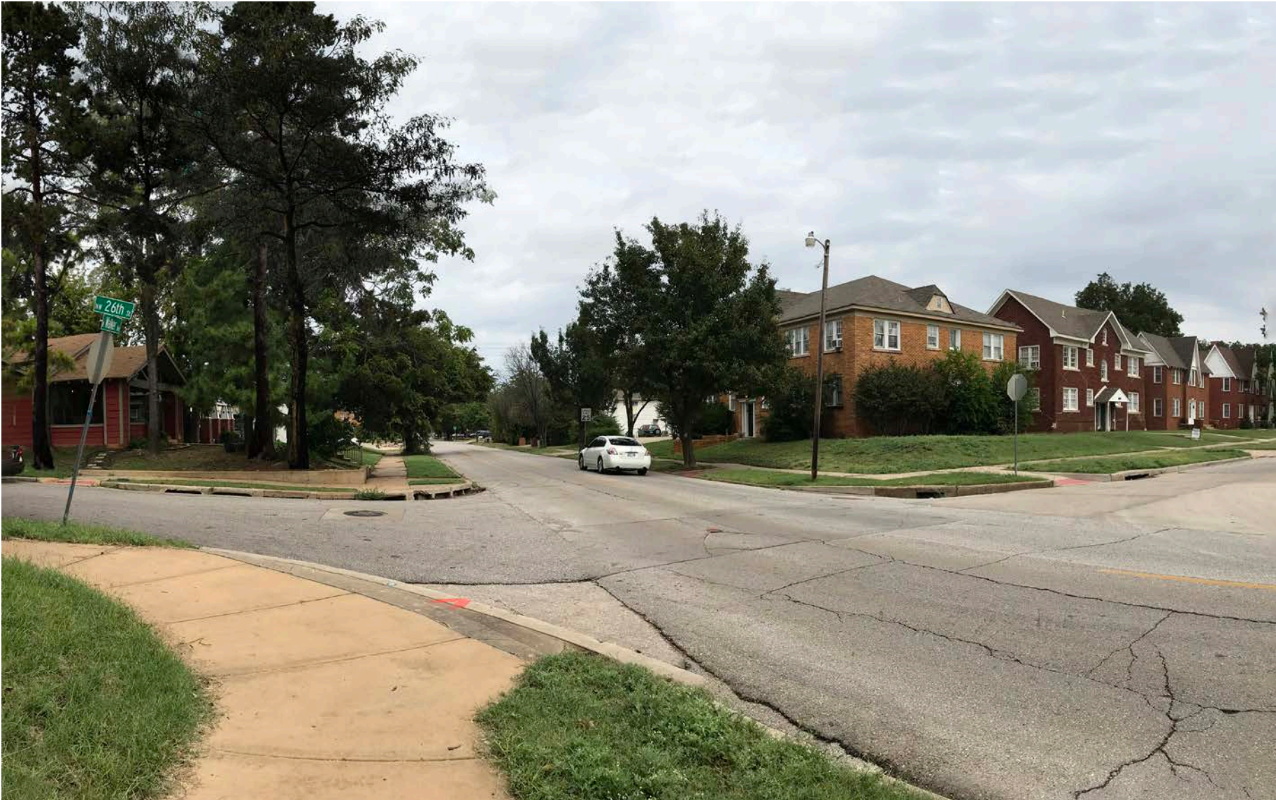
Figure 44. The large storm drains at the intersection of Walker Avenue and NW 28th Street create dangerous drops for pedestrians.
