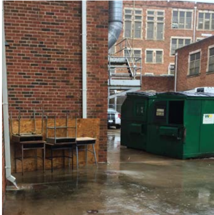
Figure 12. Rainwater from the school roof flows into the paved courtyard and contributes to flooding inside and outside the building.
