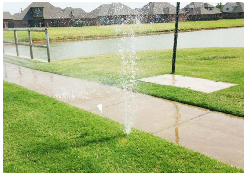
Figure 21: Broken sprinkler head found at a neighborhood association checkup
