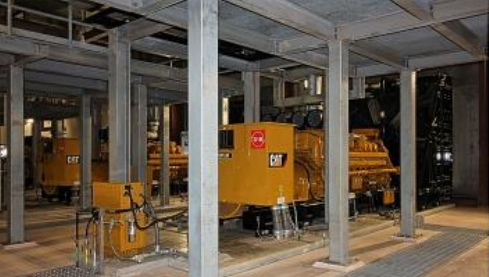
The Draper Water Treatment Plant was knocked off-line during the May 2013 tornado resulting in residents and businesses being unable to use water as crews worked to restore electricity to the plant. Emergency Generators, funded by Federal Disaster Recovery Grants, were installed at the plant to ensure uninterrupted water service in the future.
