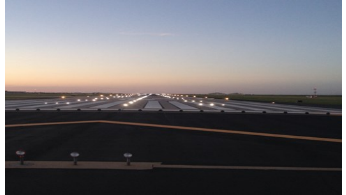
Airport Lighting Control and Movement System
