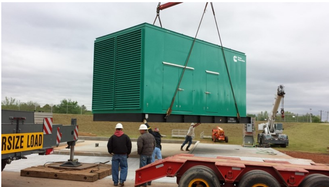
Witcher Lift Station Generator
