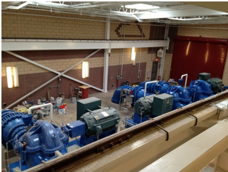
Booster pump station No. 25
