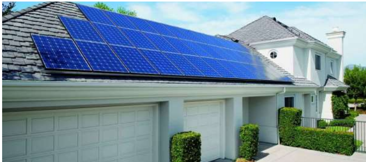
An Oklahoma City home outfitted with a photovoltaic solar array.
