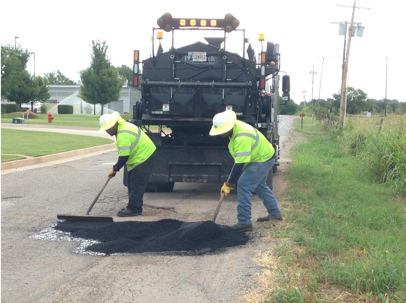
Asphalt Spread in Pothole
