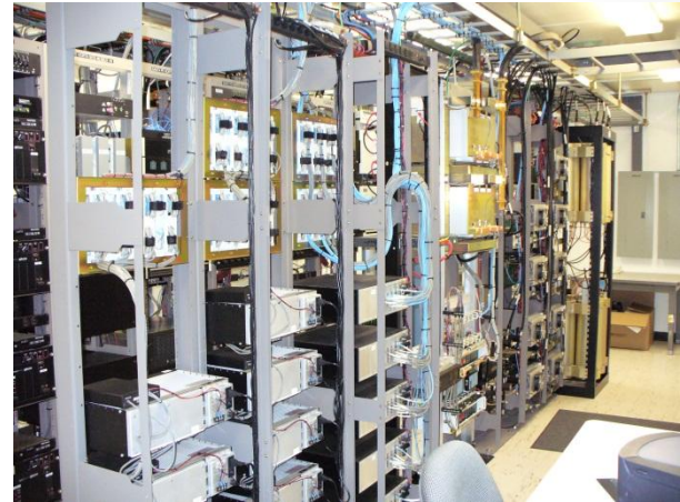
Radio System Infrastructure
