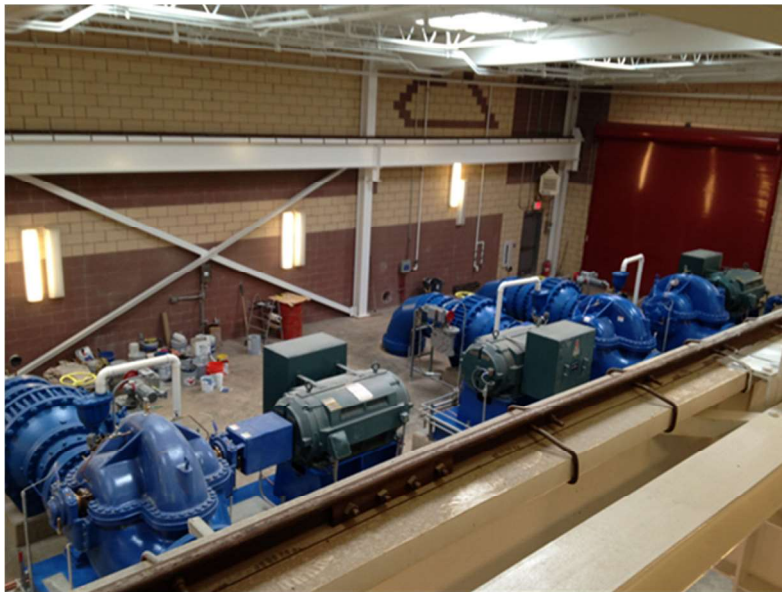
Booster pump station No. 25
