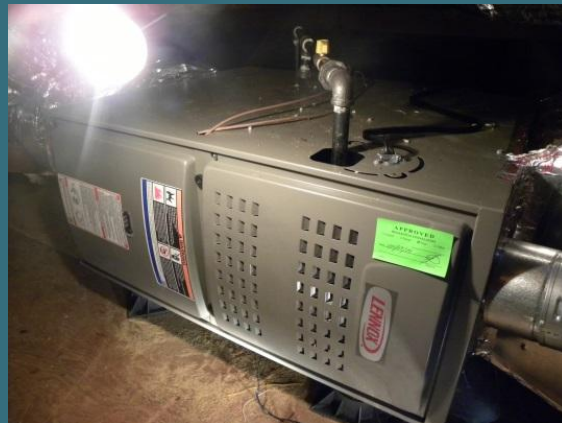
Central heat system
