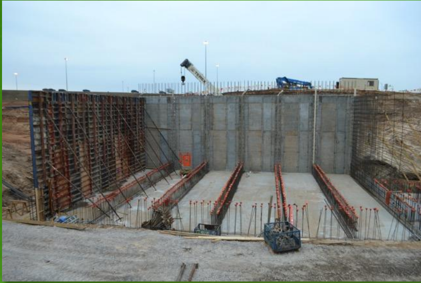
Pump Station- January 14, 2015
