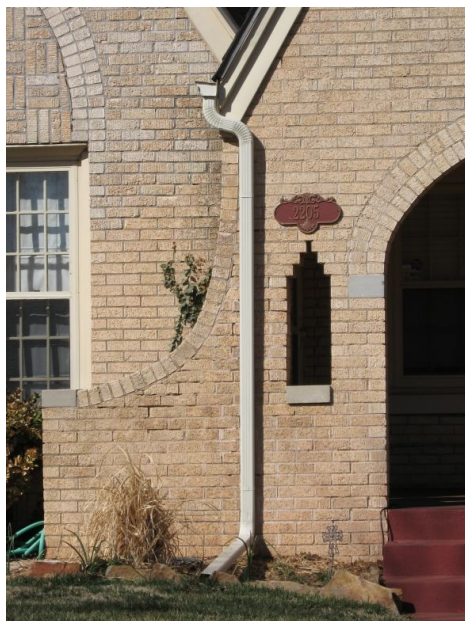
Downspouts should be located and designed to channel water away from the building (2205 NW 26th Street).
