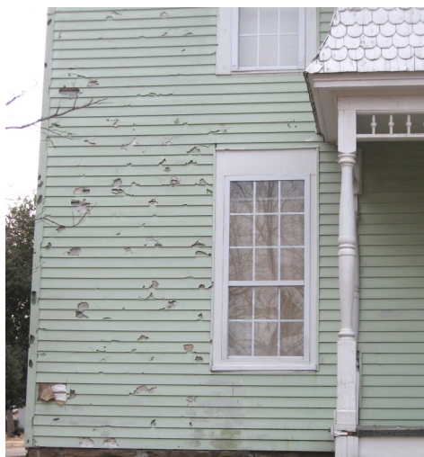
Vinyl siding is easily damaged and cannot be
