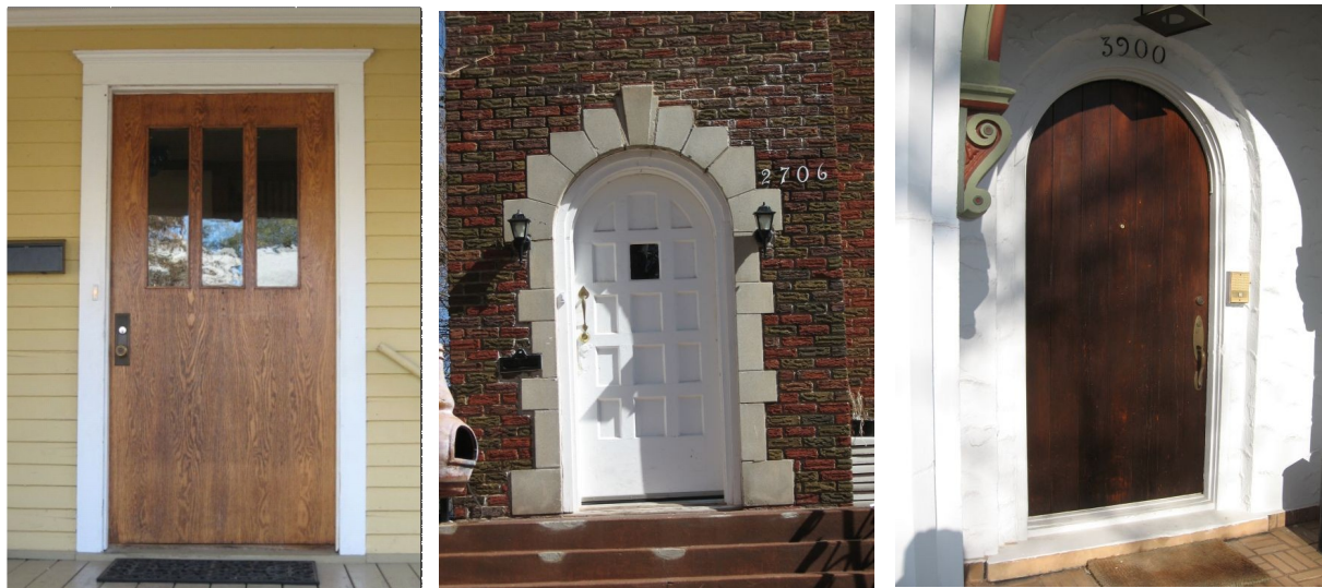
Character-defining doors: Craftsman style at 912 NW 16th Street, left; arched Tudor Revival style at 2706 Robinson, center; arched Spanish Colonial Revival style at 3900 McKinley Avenue, right.
