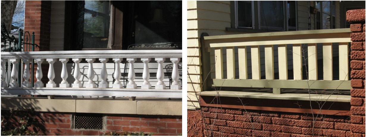
Original porch balusters (609 NW 14th Street, left, and 712 NW 24th Street, right) are character-defining and should be preserved and maintained.
