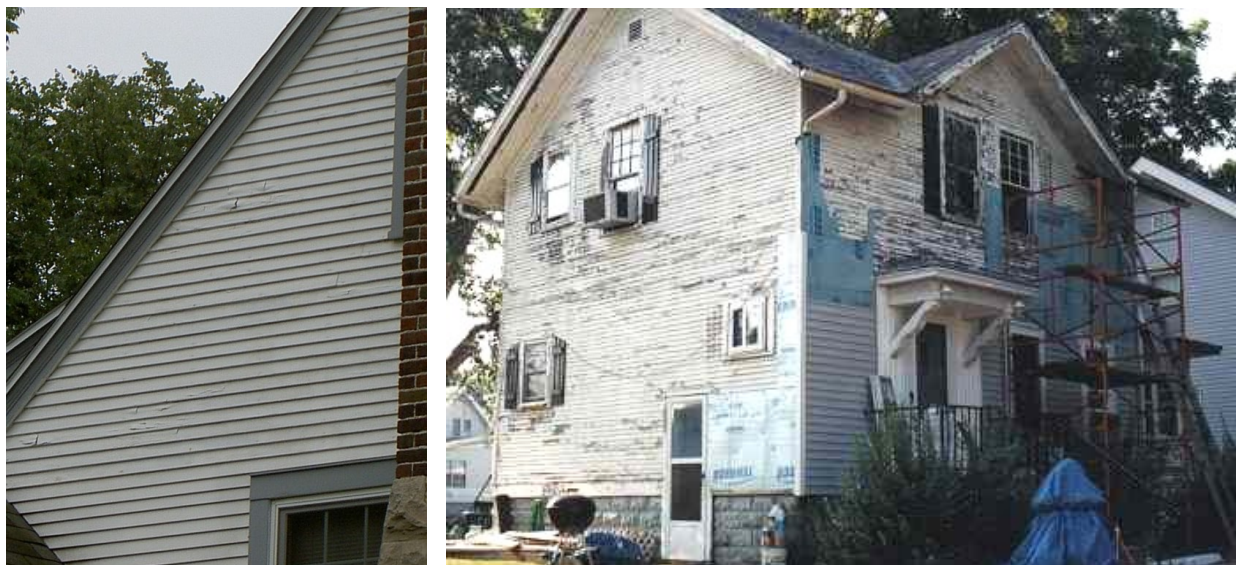
The application of vinyl siding does not allow for proper breathability of a frame dwelling and is not a sustainable material (left). After only two years, the applied polymer coating on this dwelling is already peeling (right) and the life expectancy of these materials is questionable.
