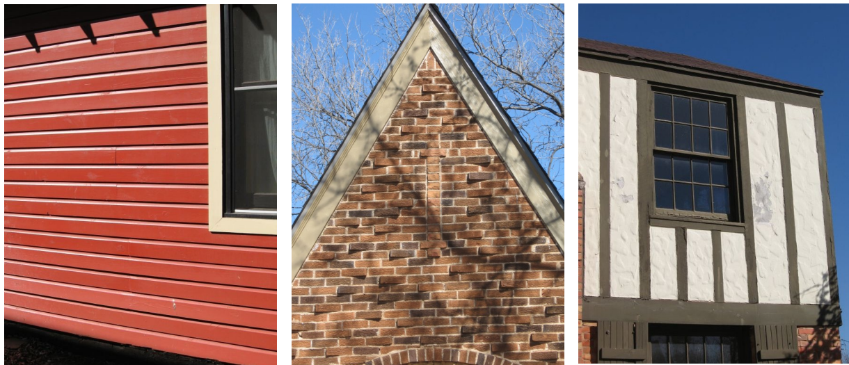
Oklahoma City's historic districts display a wide variety of original materials such as wood siding (left, 618 NW 26th Street); textured brick (center, 217 NW 31st Street); stucco and half-timbering (right, 904 NW 37th Street).
