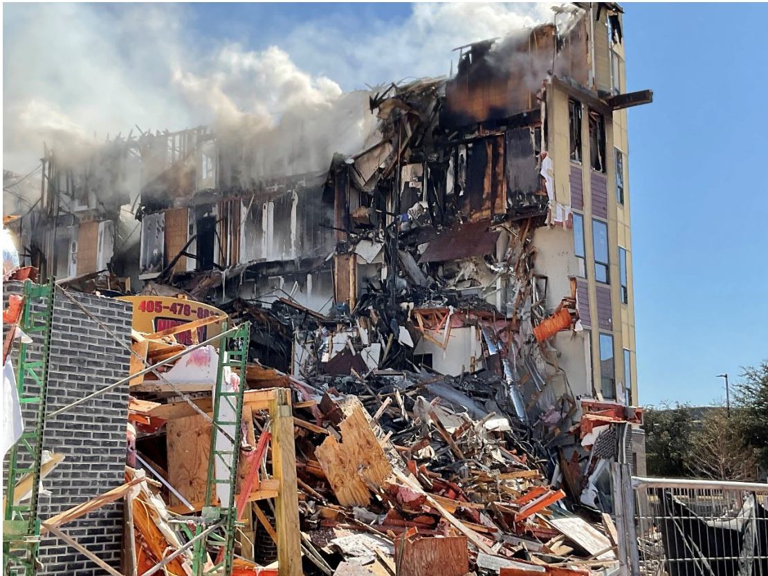
Photo taken with city issued iPhone. Picture of southwest area facing southeast.
