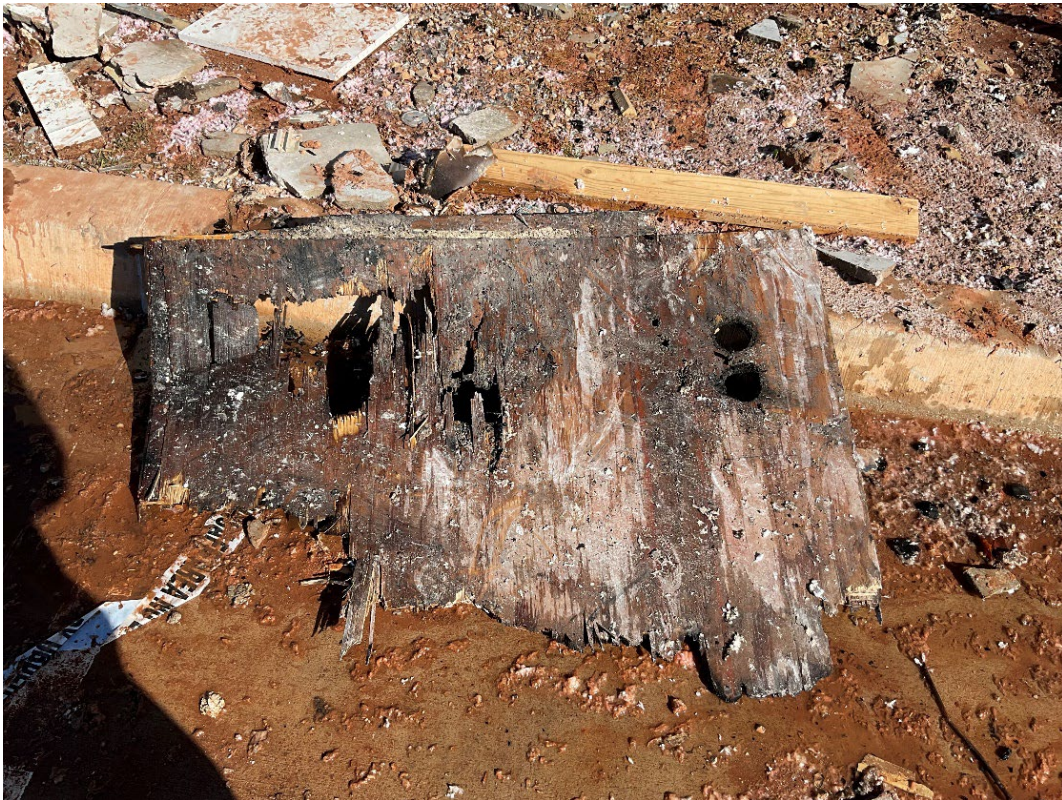
Top of flooring from 4 th floor electrical room; southwest area of building
