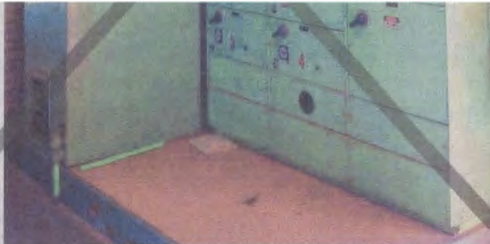
Photo 2 - PS #7 Electrical Gear
