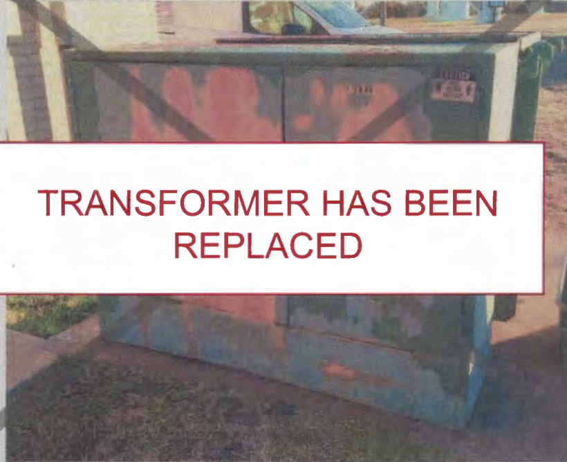
Photo 12 - PS #18 Utility Transformer
