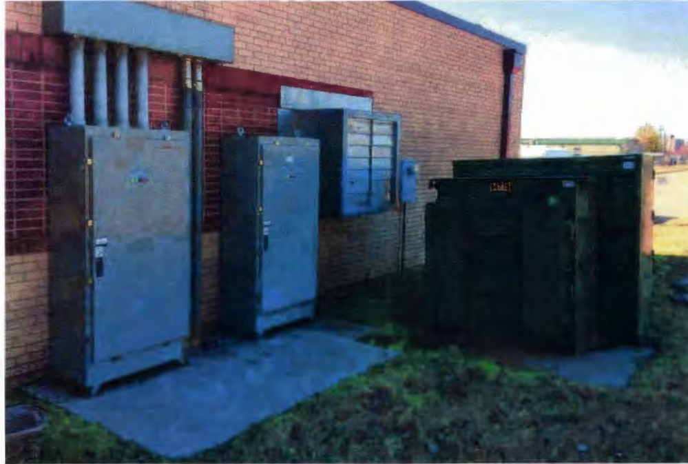
Photo 10 - PS #15 Service-Entrance Equipment
