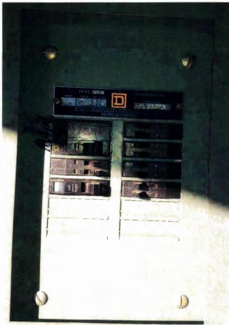
Photo 8 - PS #12 Lighting Panel
