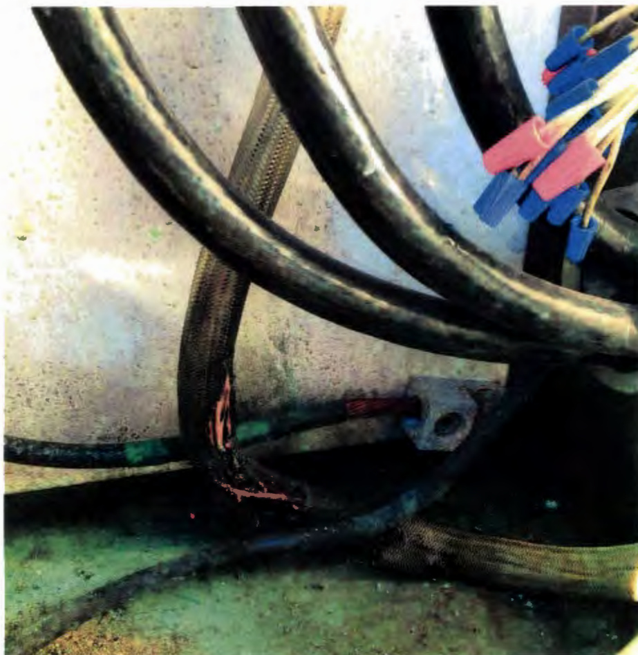
Photo 17 - PS #23 MTS with Damaged Control Wiring
