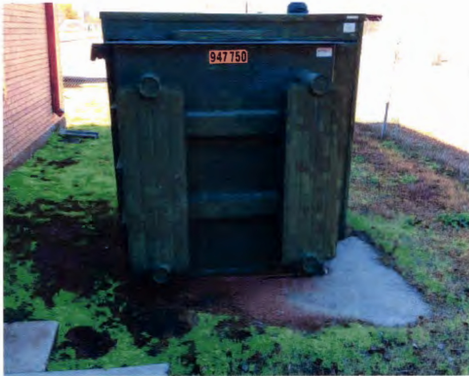
Photo 11 - PS #15 Utility Transformer
