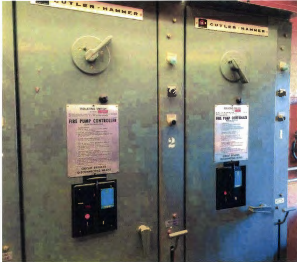
Photo 6 - PS #11 Fire Pump Starters
