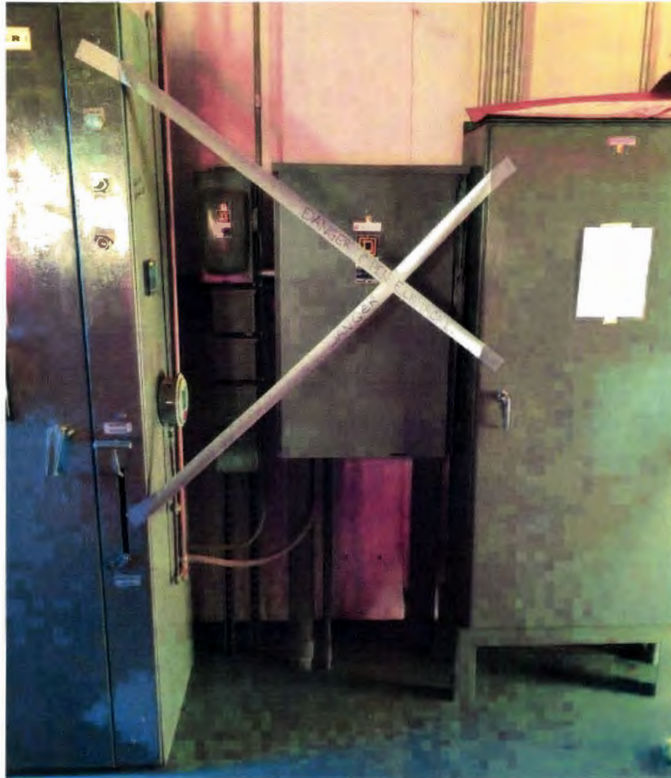
Photo 7 - PS #12 Main Disconnect
