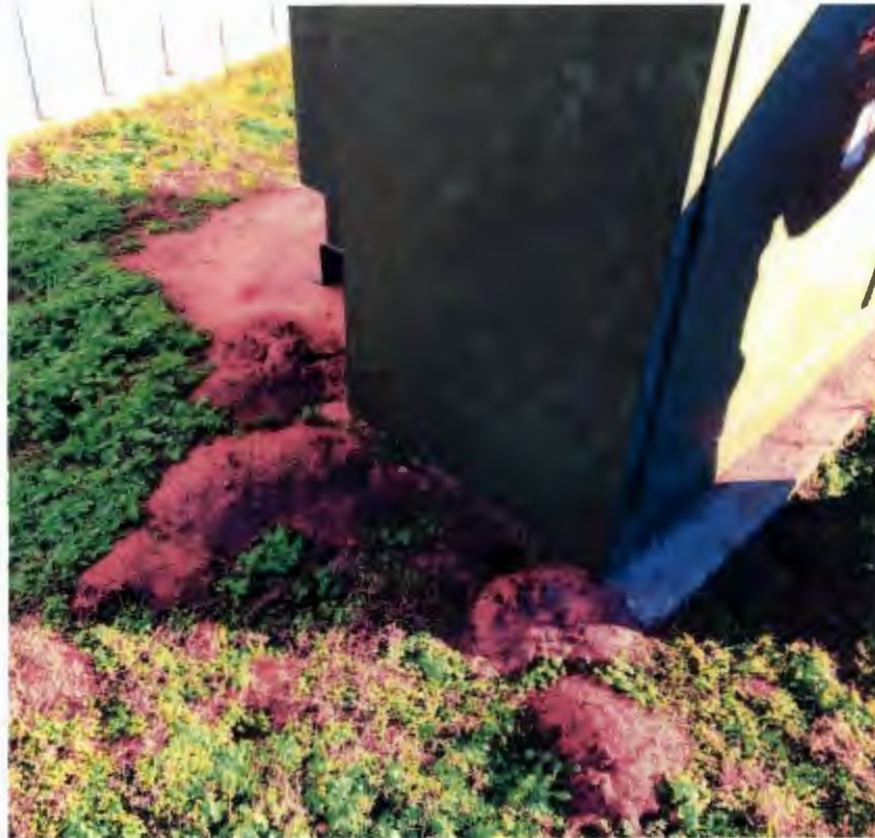
Photo 9 - PS #12 Utility Transformer
