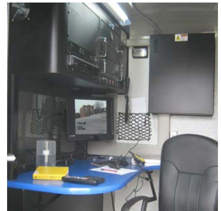
Storm drain camera systems control room
