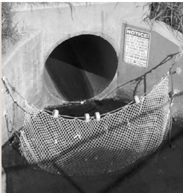
Floatable debris net
