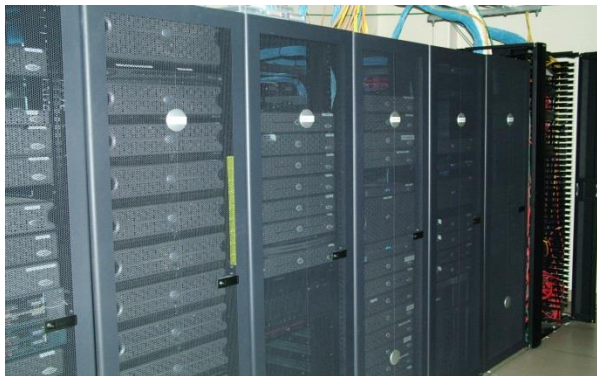
Servers and Storage
