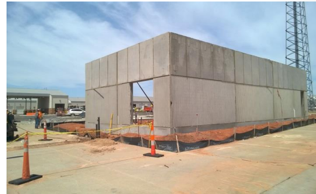
New Primary Data Center
