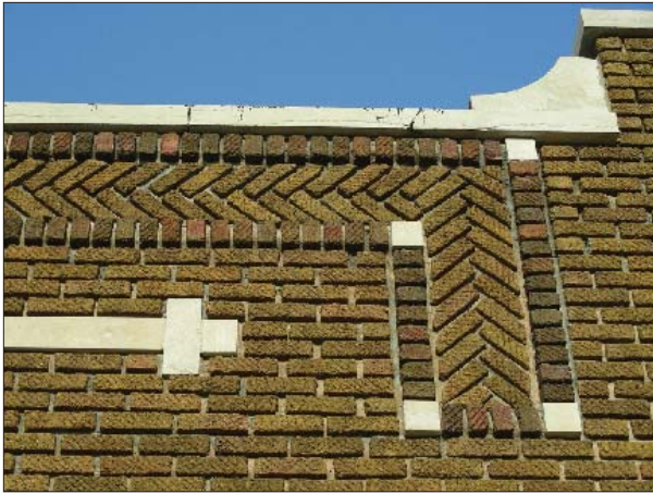
Subtle choice of brickwork tone, texture, and pattern can markedly enhance a relatively modest street facade.
