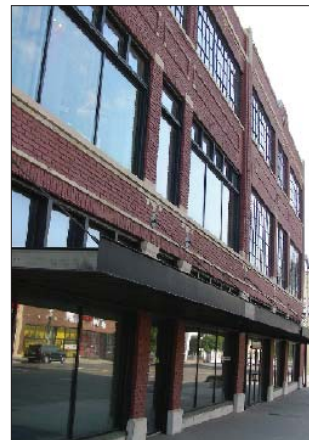
Matching original windows is usually important to the character of the building.
