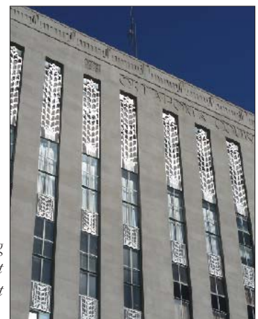
Decorative metal screening may be a significant characteristic of a street facade.
