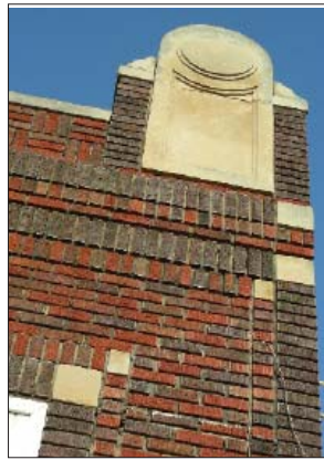
Ensure that maintenance and repair are compatible with the properties of traditional materials.
