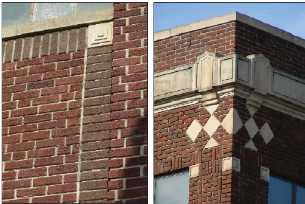
Maintain the subtlety of original detailing. Decorative brickwork, combined with contrasting masonry details, can markedly enhance a relatively modest street facade.
