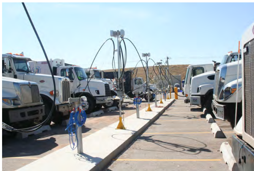
Solid Waste Management trucks refuel at the facility's slow-fill CNG fueling stations.
