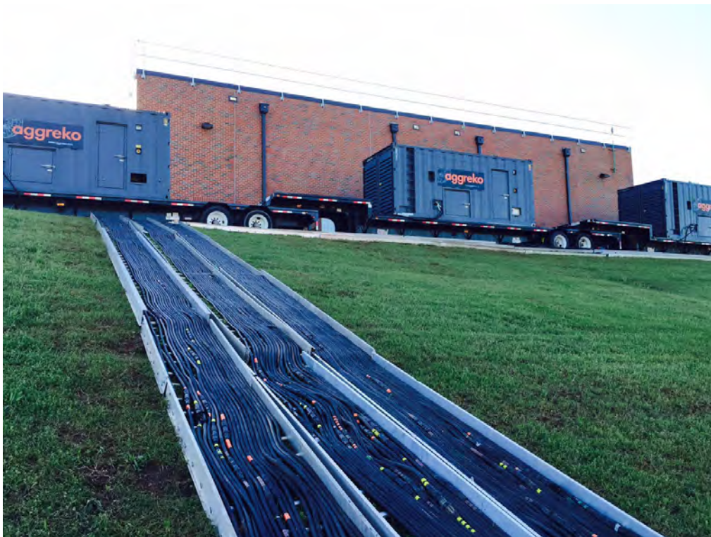
Three temporary diesel generators provide power to the Draper water treatment plant via 600 feet of cable.
