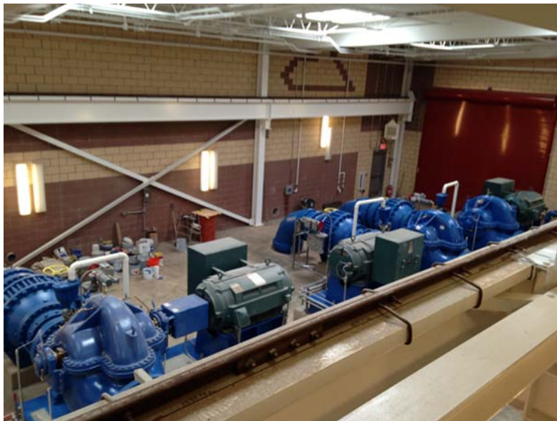
Booster pump station No. 25
