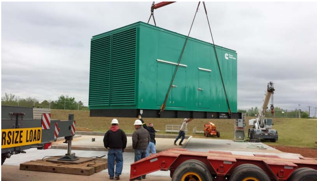
Witcher Lift Station Generator
