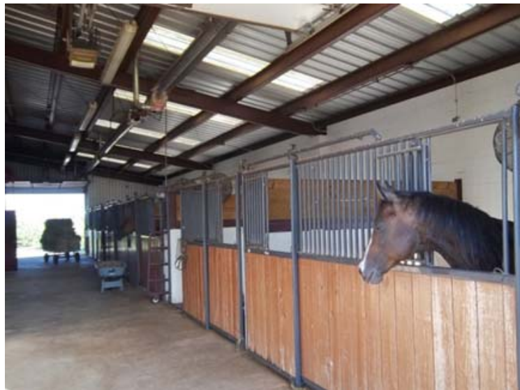
Livestock Barn Sprinkler System
