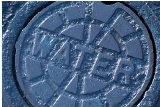
A meter tile marks access to an OKC water line.
