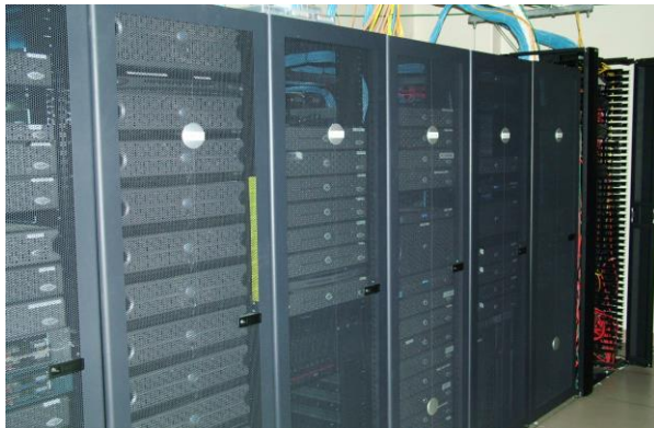
Servers and Storage
