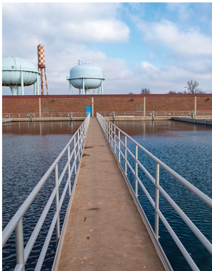
Figure 13: Draper water treatment plant
