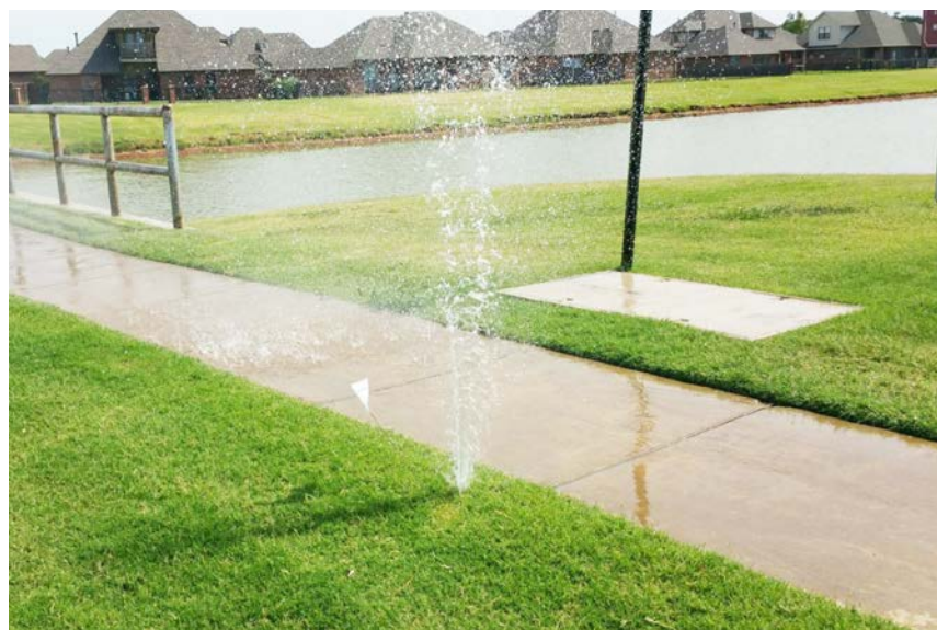
Figure 21: Broken sprinkler head found at a neighborhood association checkup
