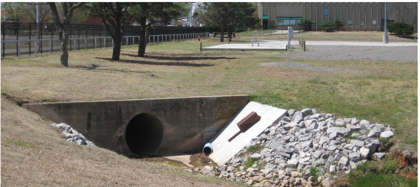
State Fair Park Sand Filtration Unit
